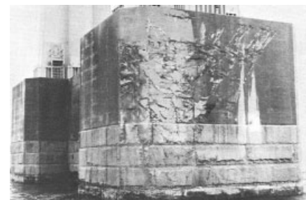
Fig. 3. Newport Bridge, RI, USA, damage to pier
