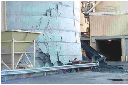
Fig. 8. View of external damage at MEA coal silo (Kazas 2001, with permission from Morgantown Energy Associates Plant)
