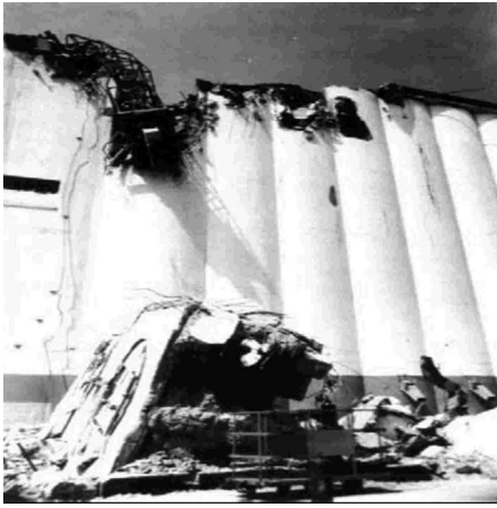
Fig. 11. Partial collapse of grain silo during 1974 Lima, Peru earthquake (USGS 1974)
